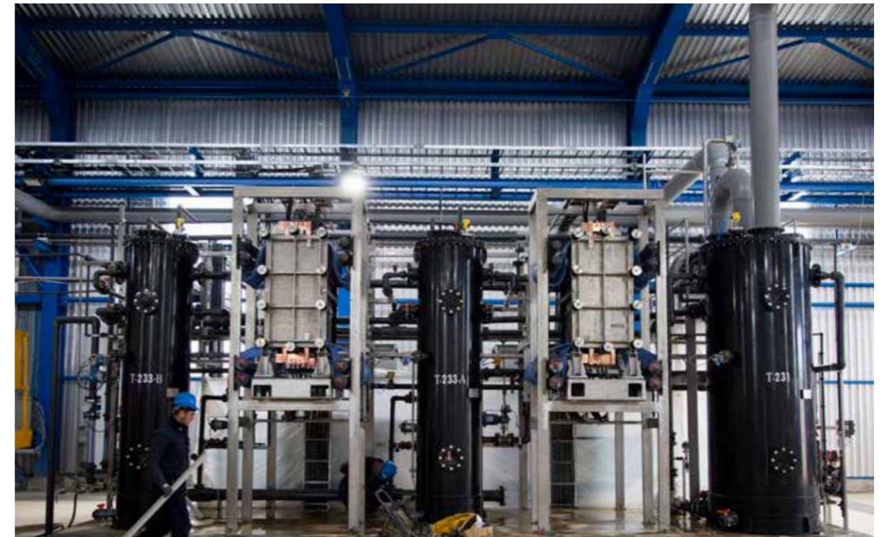
Ak-Kim Ultrafiltration Facility
