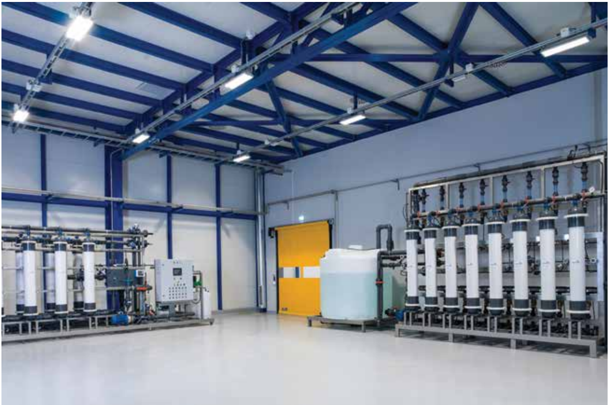
Ak-Kim Ultrafiltration Facility
